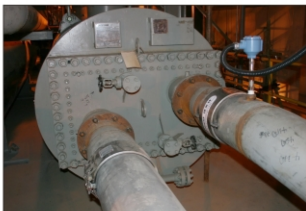
Gas making processing equipment pipe with annual production of 600 thousand in SOPO Group uses Jointand pipe joint for connection.
