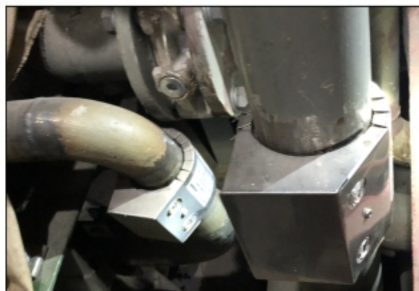
The polar luxury cruise built by China Merchants Heavy Industry uses Jointand fire-resistant pipe joint for connection.
