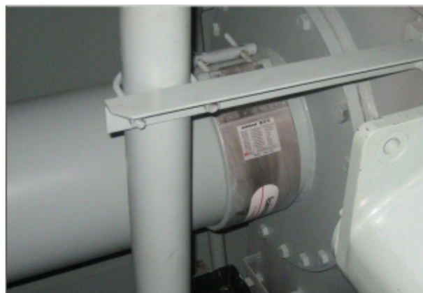
Low-speed marine diesel engine produced by Shanghai CSSC-MES uses Jointand pipe joint for connection.
