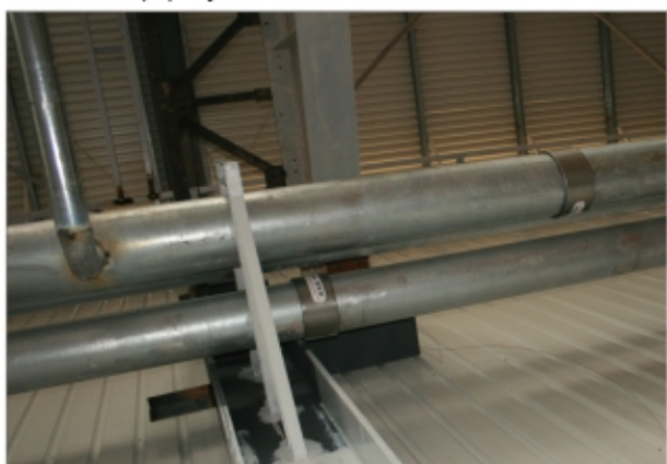
Production line process pipeline of Chongqing Changan Ford Automobile uses Jointand pipe joint for connection.
