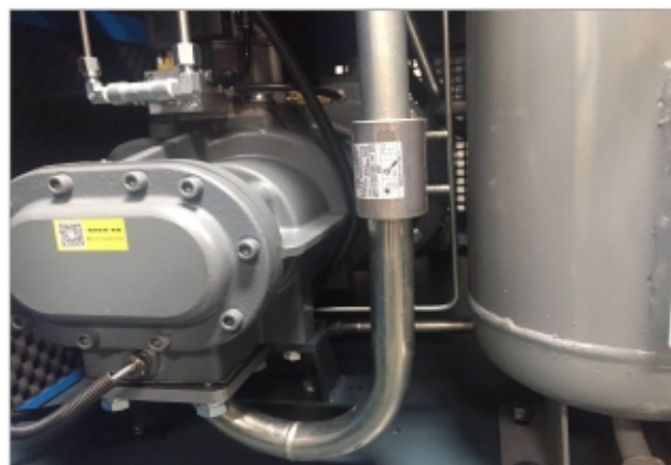
Compressor oil system pipeline uses Jointand pipe joint for connection.
