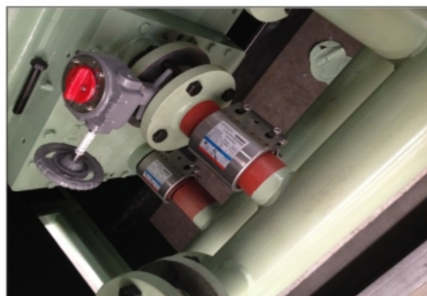
Japanese IHI compressor equipment uses Jointand GL pipe joint for connection.
