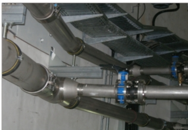
Three Gorges hydroelectric power station, annular pipeline inside unit uses Jointand pipe joint for connection.
