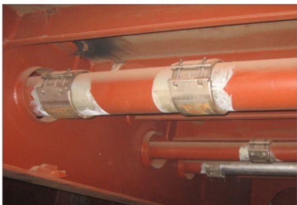
Roll-on roll-off ship built by Guangzhou Shipyard International uses Jointand pipe joint for high-temperature water system pipe connection.
