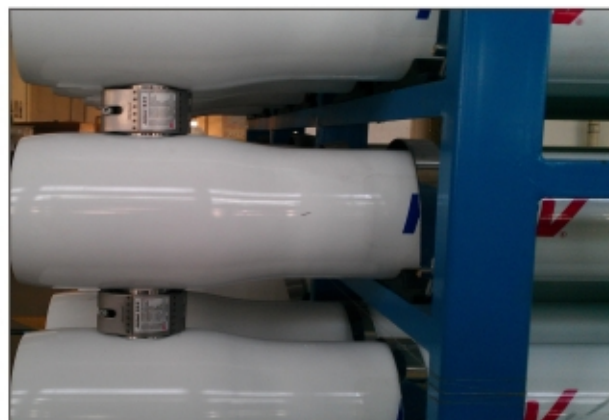
Water treatment membrane equipment uses Jointand pipe joint for connection.
