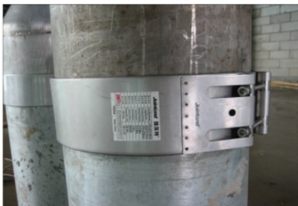
Two kinds of different metal pipelines of stainless steel pipe and carbon steel pipe in siphon system of Yangzhou Airport use Jointand pipe joint for connection.
