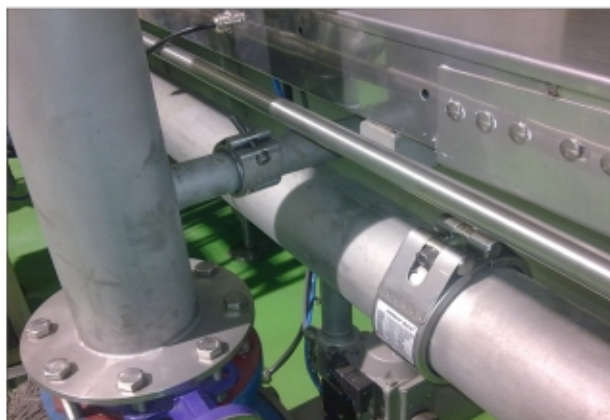
Sterilization machine equipment pipe of Kunshan Suntory uses Jointand pipe joint for connection.
