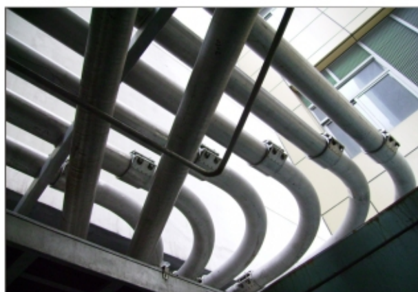
Production line process pipe connection of Wuxi LANXESS Energizing Chemistry uses Jointand pipe joint for connection.
